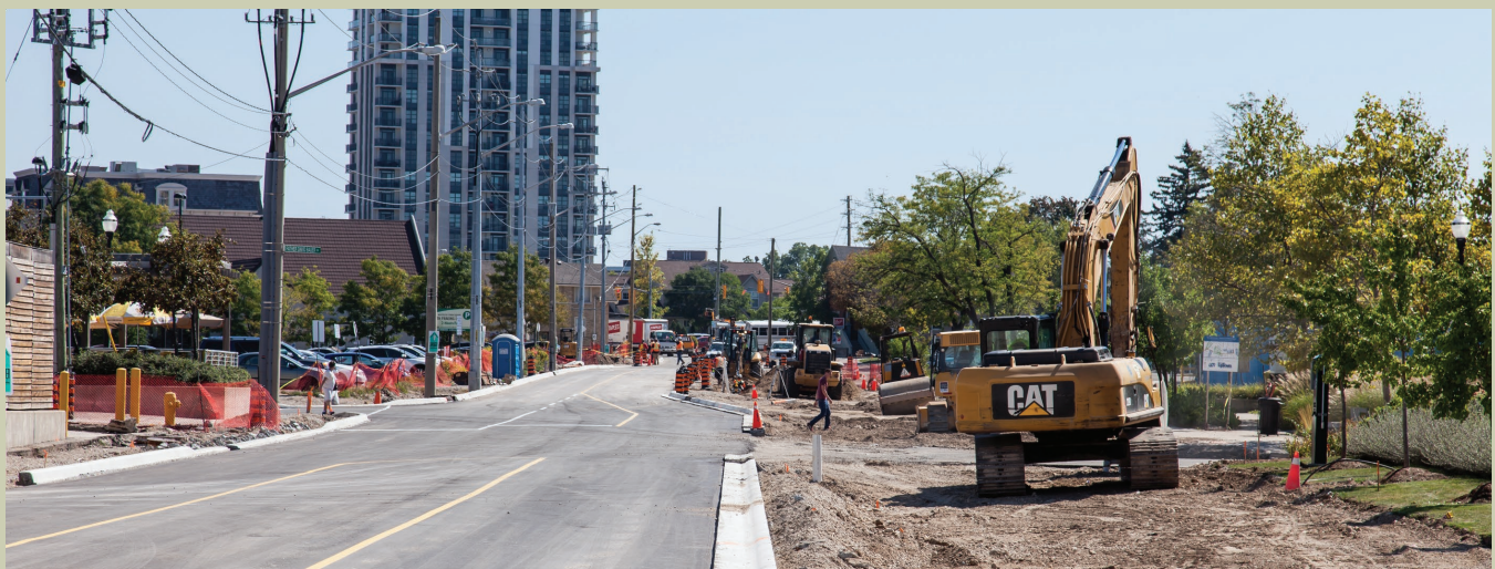
Caroline St prepared for tracks, the train will run to the right in this photo
