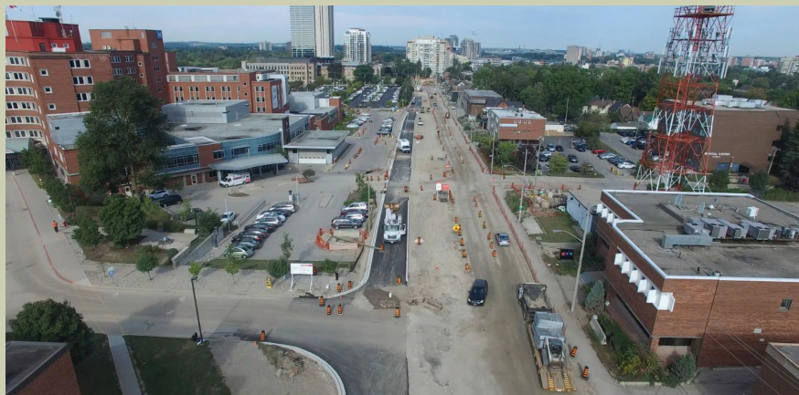
Section of King St in front of Grand River Hospital (Left) is ready for paving and track work, the train will run down the centre of King St with a traffic lane on either side
