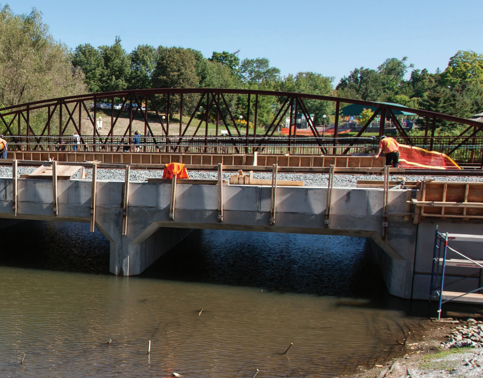
A series of culverts create a crossing over Laurel Creek in Waterloo Park, the former crossing was an aging wooden structure
