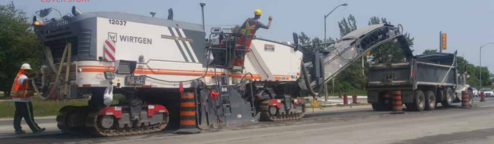
Added benefit: 3D milling allows for the adjusting of forecasted recycled asphalt production, trucking and storage for each job.
