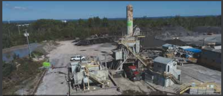
GREEN INFRASTRUCTURE PARTNERS (GIP) INC. Bearbrook Asphalt Plant
