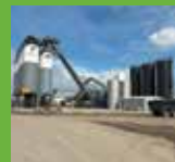
THE MILLER GROUP Pave-AI Asphalt Plant #26
