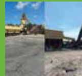
THE MILLER GROUP North Bay Asphalt Plant #13
