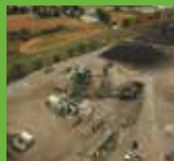
STEED AND EVANS LIMITED Kitchener Asphalt Plant
